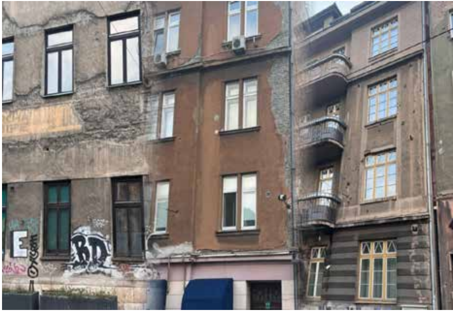
Figure 3. Houses with bullet holes near Baščaršija, Sarajevo
